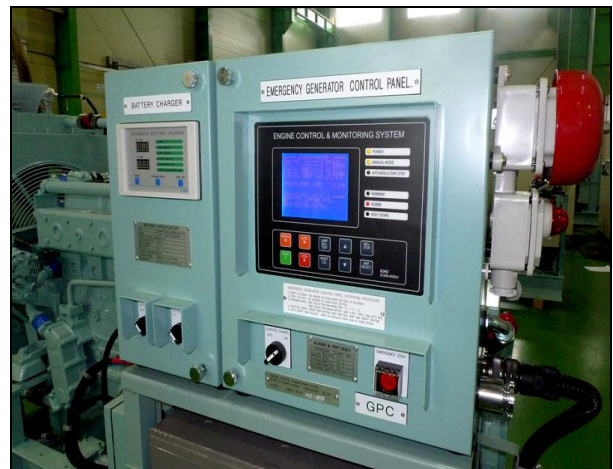
Digital Type Control Panel
