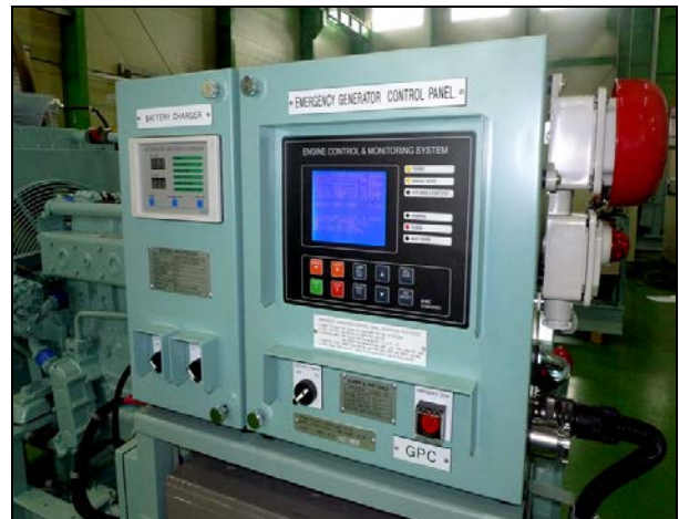
Digital Type Control Panel
